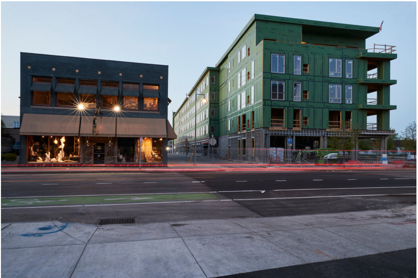
A new apartment building under construction, next to a florist and interior design shop that sat atop the highway for decades. Mustafa Hussain for The New York Times
